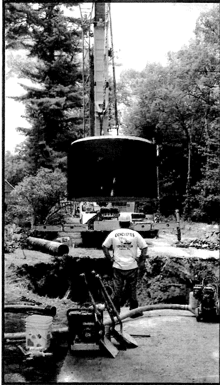
Photo 3 - Installation of the lower section of the precast concrete Contech CDS 4030 Stormwater Treatment Unit.
